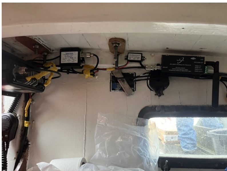
AIS installation. Wiring to be desired..!
